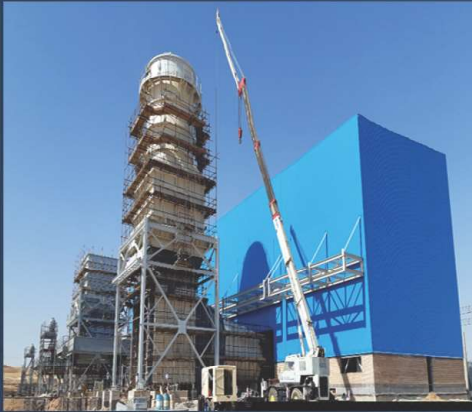
ARIAN, 546 MW C. C. Power Plant
