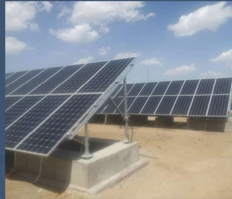
TAKESTAN, 1 MW Solar Farm
